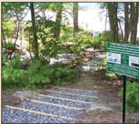
The LCC crew at Lake Waukewan designed and installed this set of infiltration steps in response to a request from the property owner.
